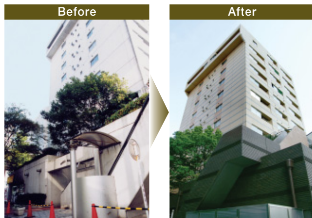
Completed in 1981, THE Palms Gotanda in Shinagawa Ward was restored to newly built condition through complete renovation of all common areas, including facades, entrance and exterior.
