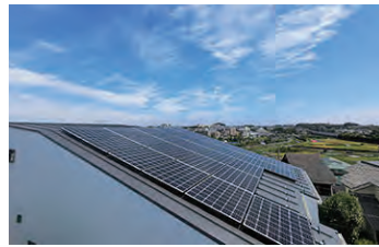
Solar power generation system
