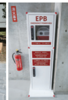
Emergency Power Box
